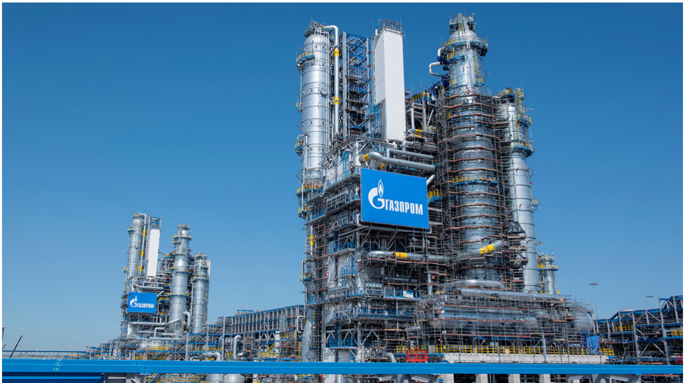
Amursk gas processing plant. Gazprom
