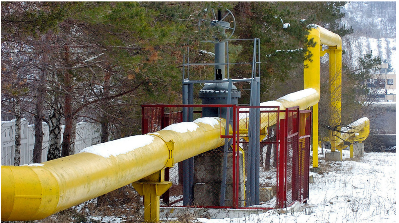
Gas distribution point of the Chisinau Thermolectric power plant. Valery Denisov / TASS
