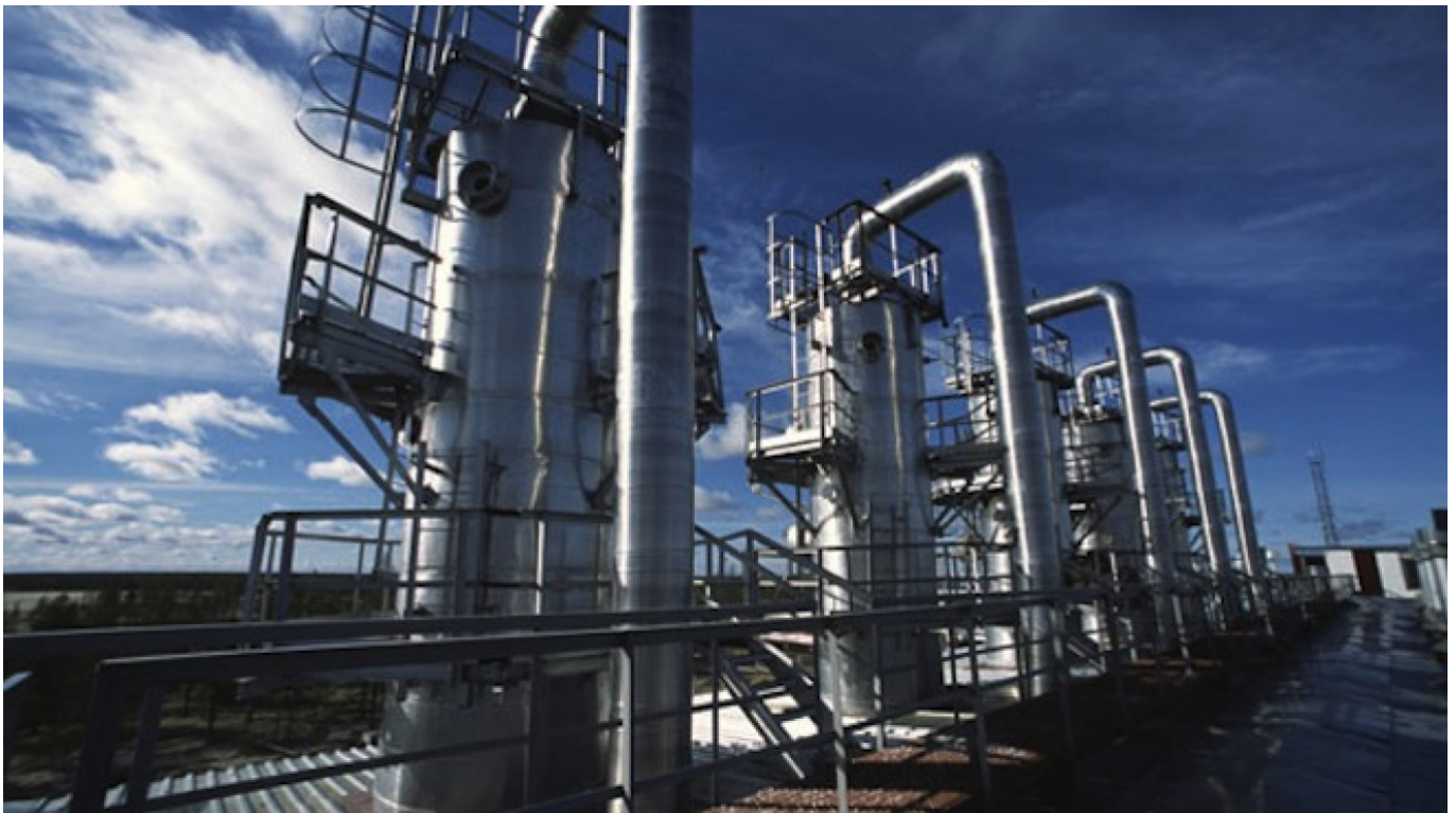
A Novatek facility
